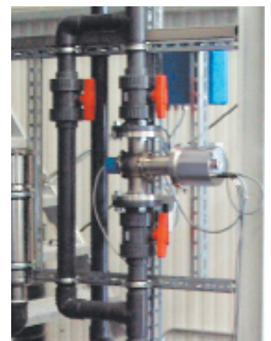
Straight pipe installation with ultrasonic cleaning system
